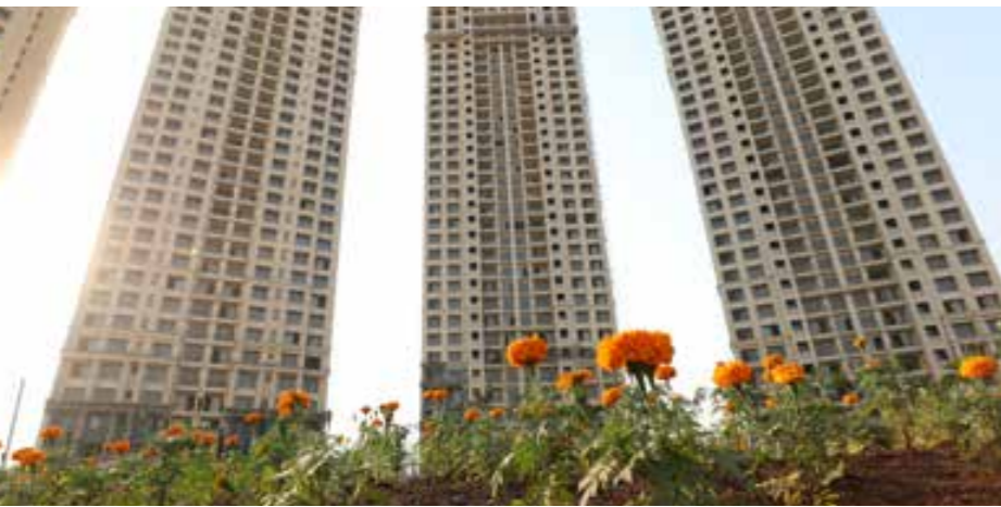
ARGUS CLIO HELIOS IN BACKGROUND: PODIUM LANDSCAPING WORK IN ADVANCED STAGES OF COMPLETION
