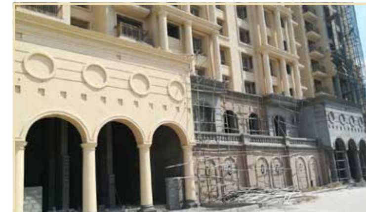
The Highlands South, Chartwell I & II: Entrance porch construction work in progress
