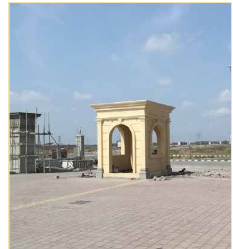
The Highlands (High Rise Buildings) - South: Retail zone security cabin and entrance gate construction in progress
