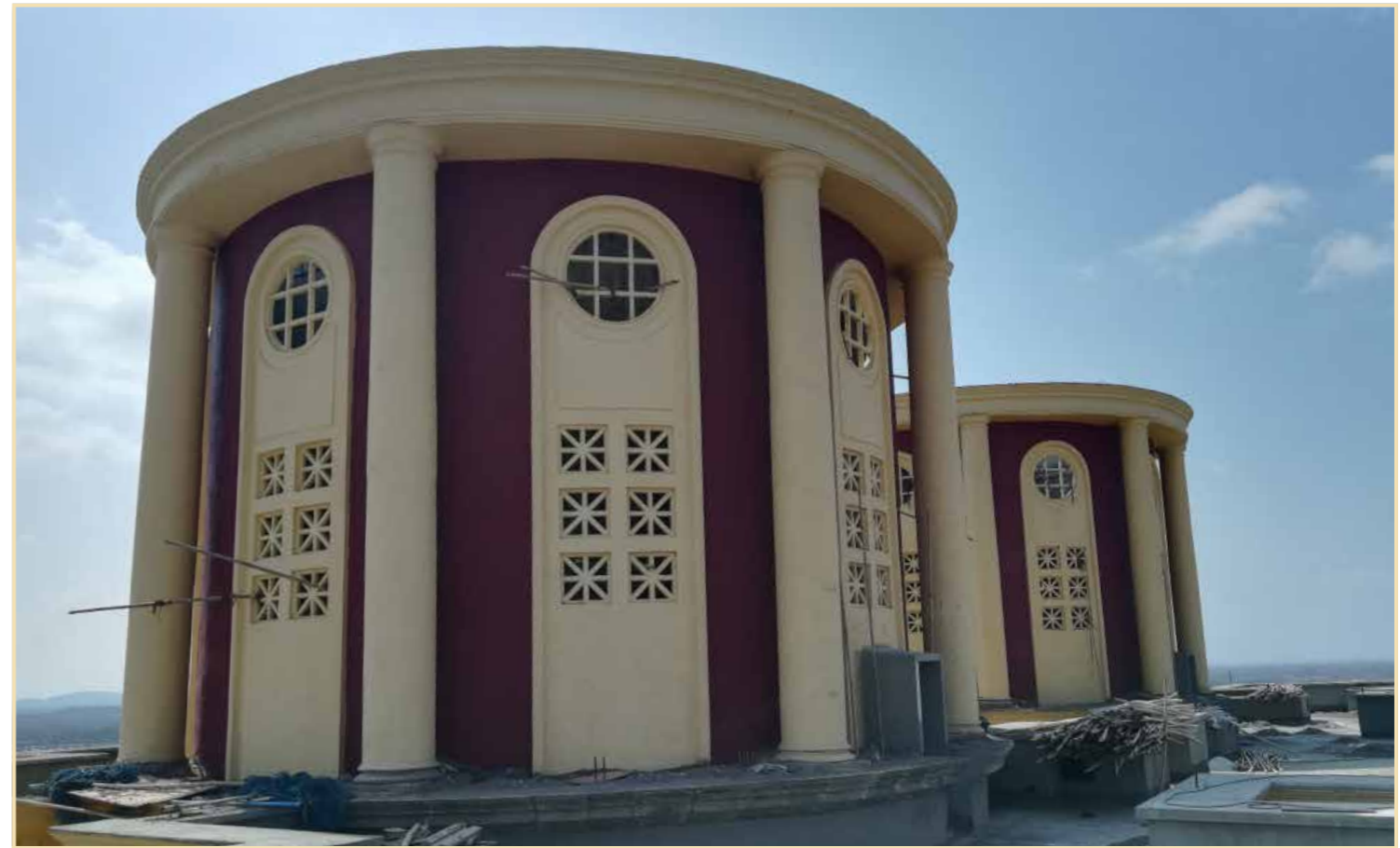
The Highlands South, Clarendon I & II: Lift maintenance room and terrace finishing work in progress
