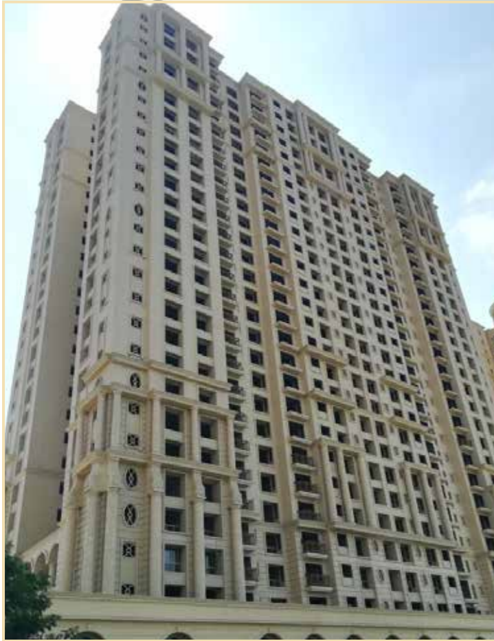
The Highlands South, Chatsworth I & II: Front facade finishing work in progress
