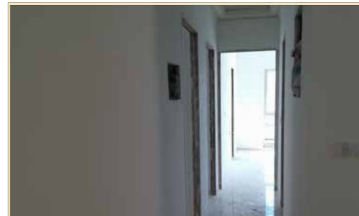
The Highlands South, Chartwell I & II: Internal flat finishing work in progress
