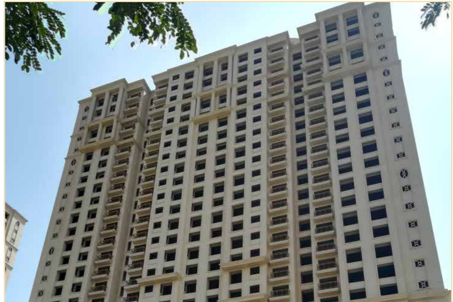
The Highlands South, Clarendon I & II: Front facade finishing work in progress
