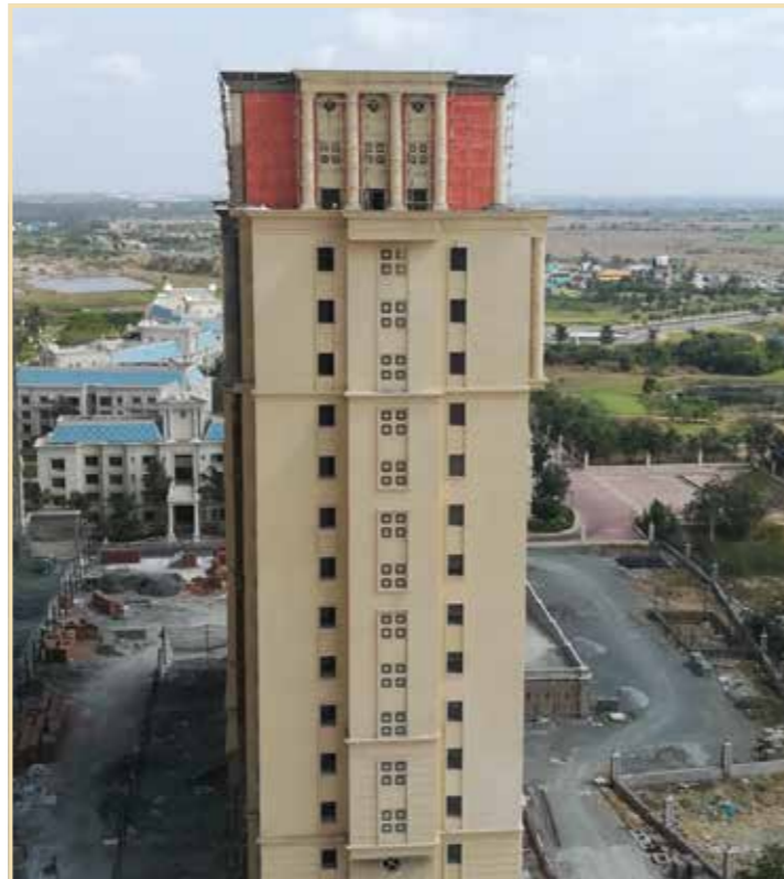
The Highlands South, Warwick I & II: Lift maintenance room and terrace finishing work in progress
