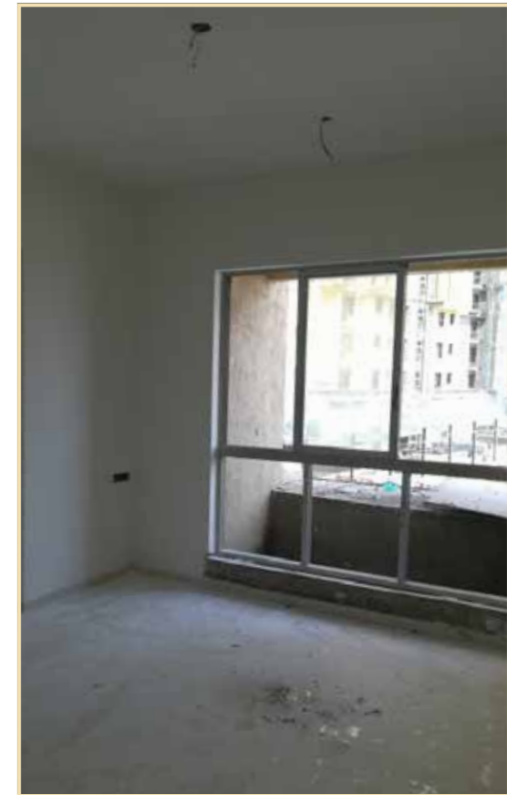
The Highlands South, Chartwell I & II: Internal flat finishing work in progress
