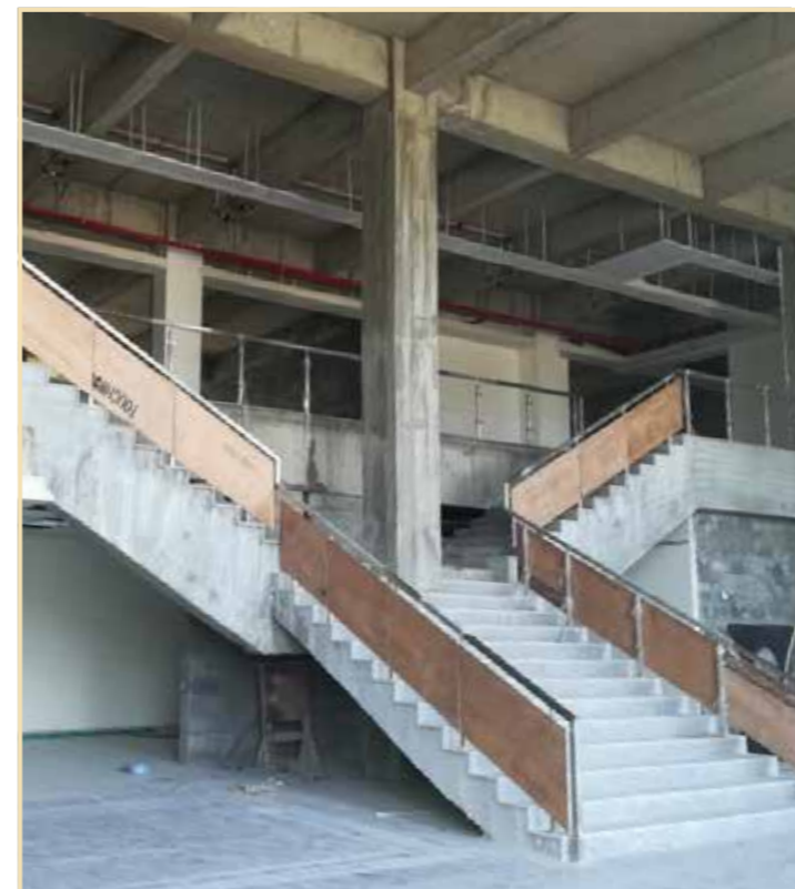
The Highlands (High Rise Buildings) - South: Retail zone lobby work in progress
