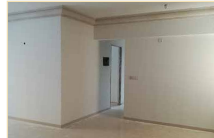
The Highlands South, Chartwell I & II: Internal flat finishing work in progress
