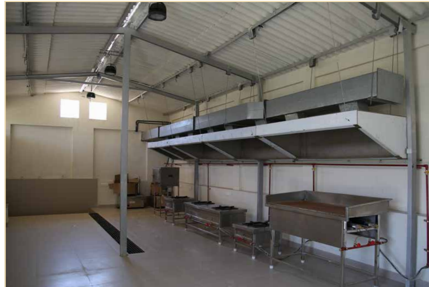
Main kitchen at Thriveni Auditorium
