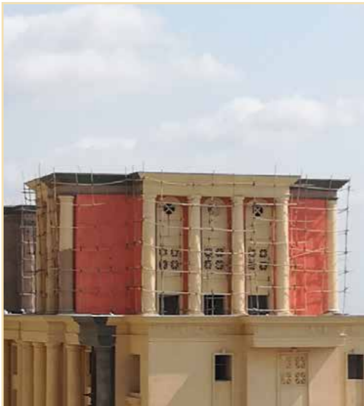
The Highlands South, Warwick I & II: Lift maintenance room and terrace finishing work in progress
