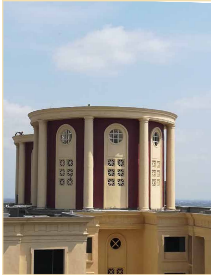
The Highlands South, Chatsworth I & II: Life maintenance room and finishing work in progress
