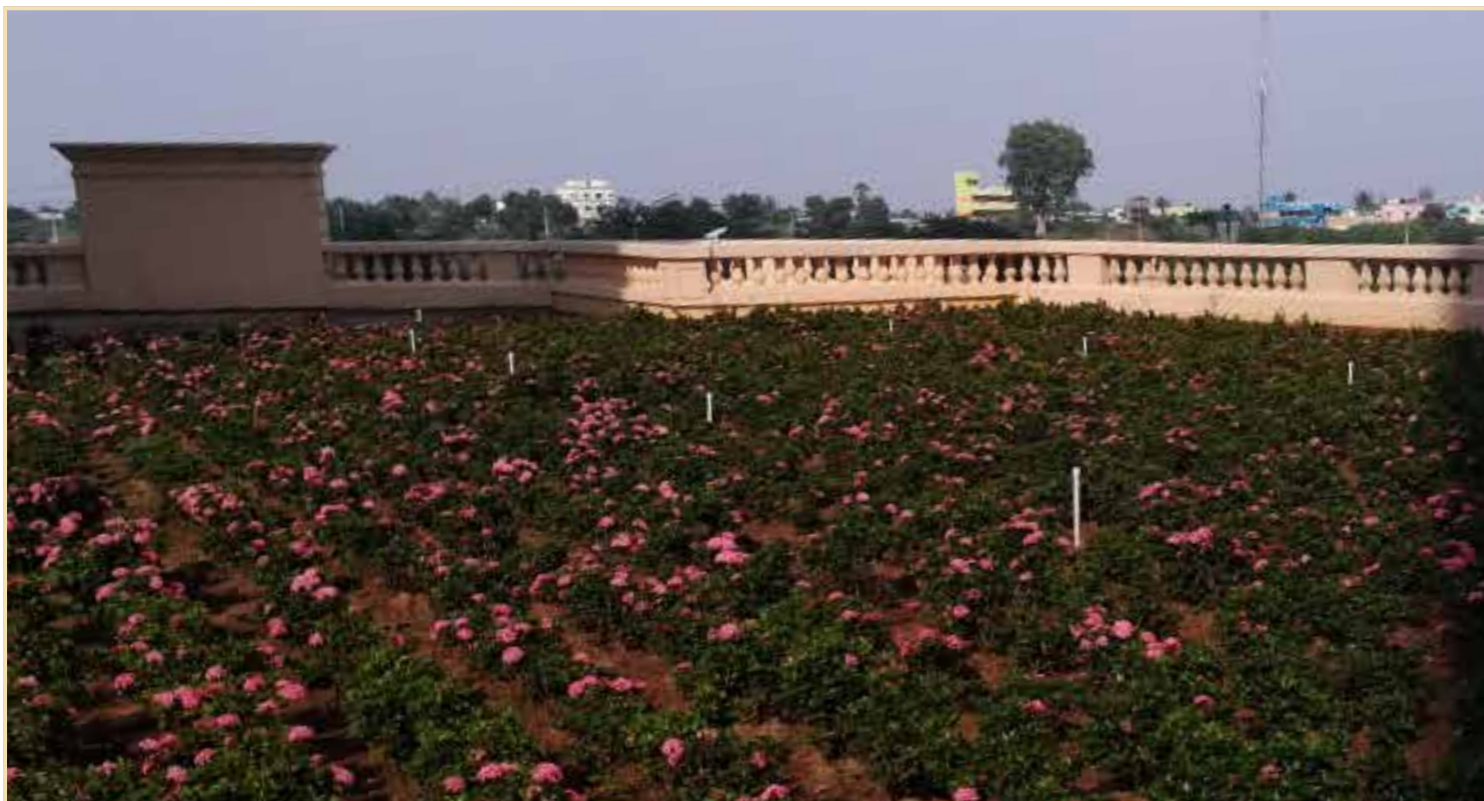
The Highlands (High Rise Buildings) - North: Podium horticulture & beautification work in progress
